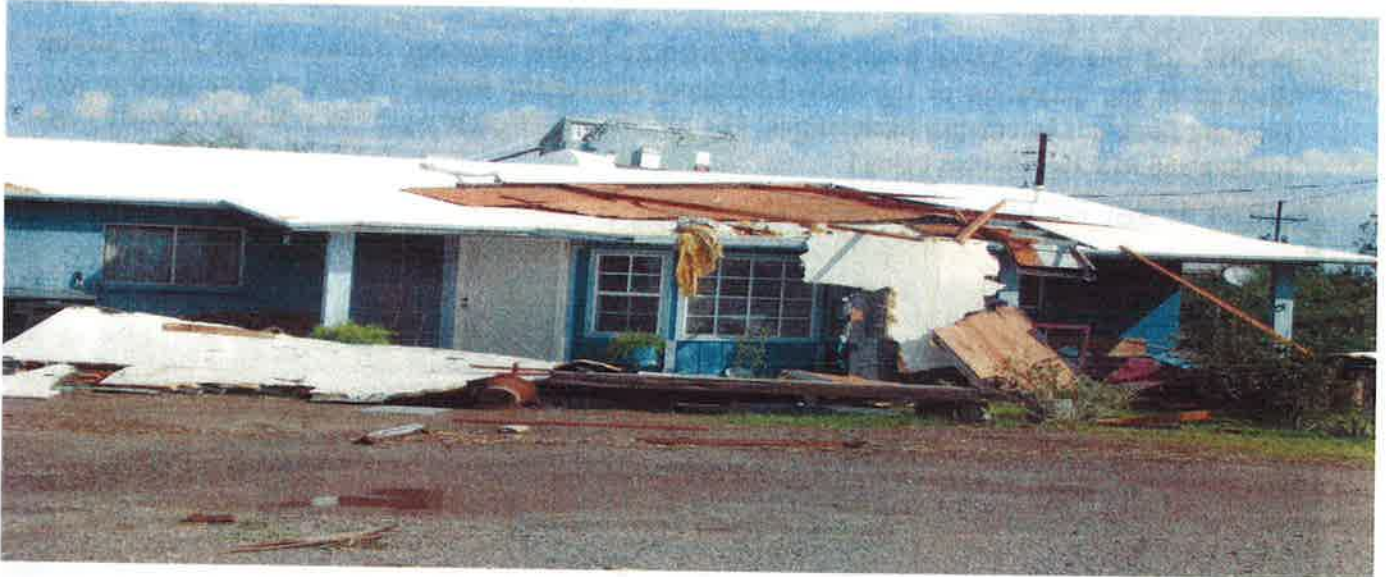
District 1-Damaged Home from August 14, 2012 Thunderstorm
